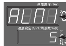
warning of temperature control irregularity 1 type: correspond to thermocouples of outlet of device.
